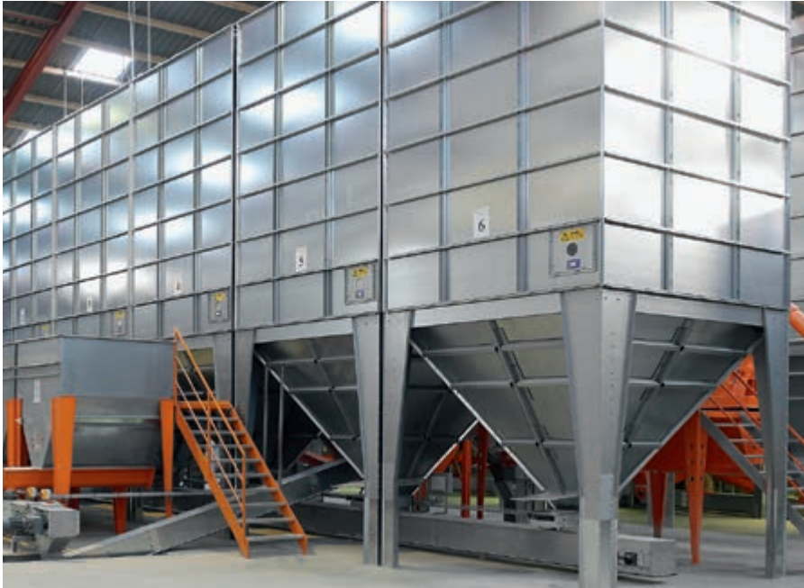
Indoor silos for storage of completed mixes
